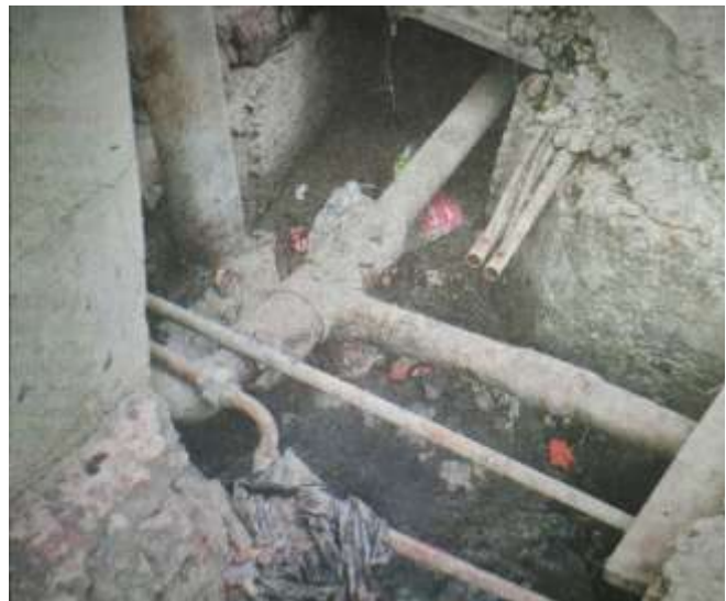
Fig.: 10 Rusty pipeline passing through the drainage
