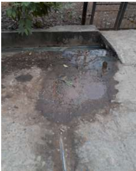
Fig.: 9 leakage of supply pipeline
